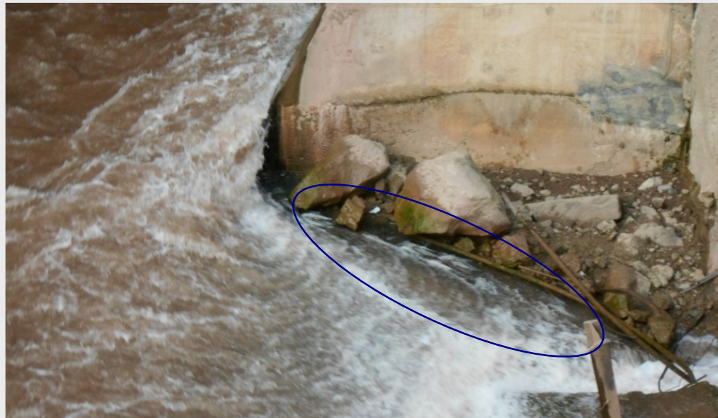
Fish Entrapped at the Mouth of Tunnel
